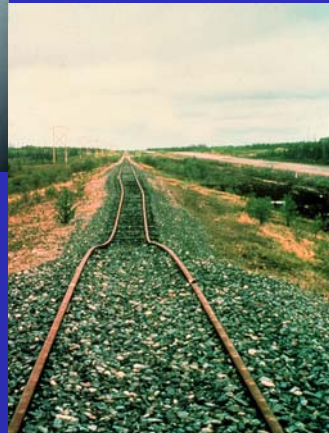
Damage to buildings and infrastructure
