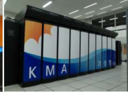
Phase 2 Cray XE6 Systems (one system in each hall)
